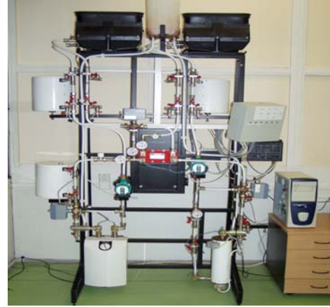
Fig.3. A photograph of the laboratory heating system
